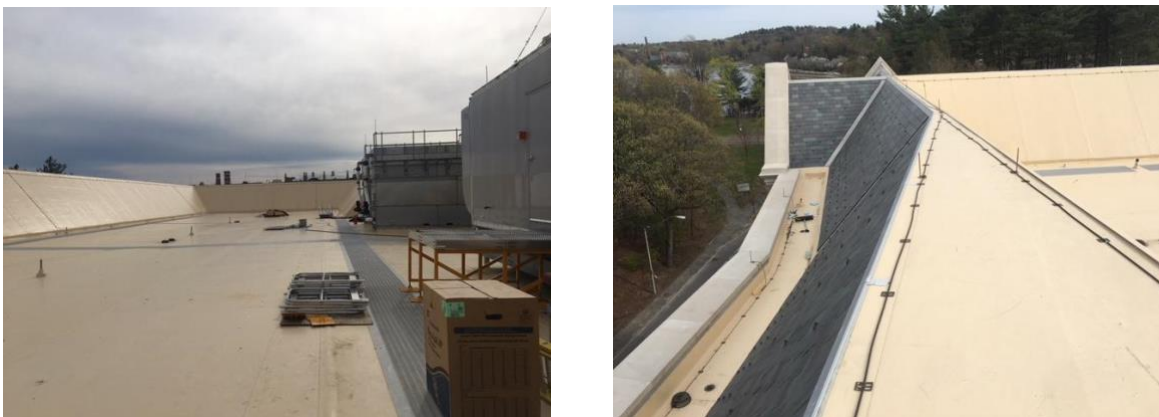
Figure 14 & 15: Pictures of the potential roof space, showing the height of the perimeter and the flat roof surface.
